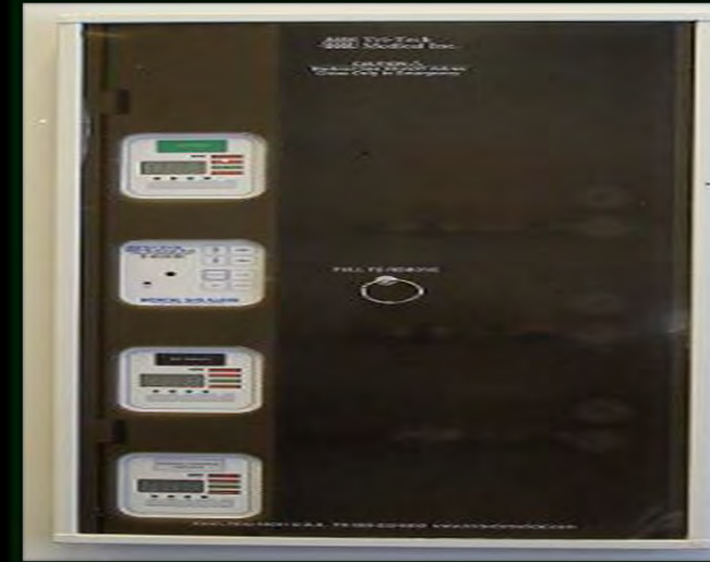
Vertical Zone Valves Box
