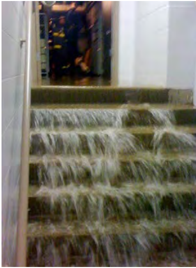
Broken pipe in CSP
